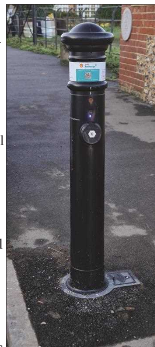
EV charging point
